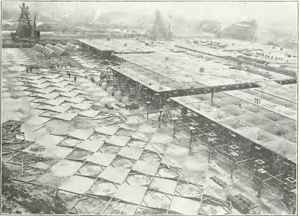
FILTER BEDS Pittsburgh Filtration Plant
